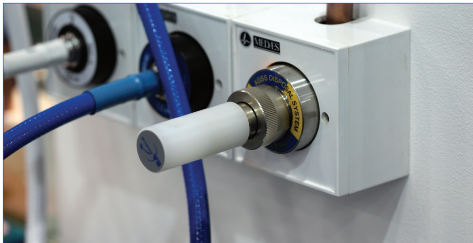
Figure 3. Centralised anaesthetic gas scavenging system used in hospitals and large clinics
